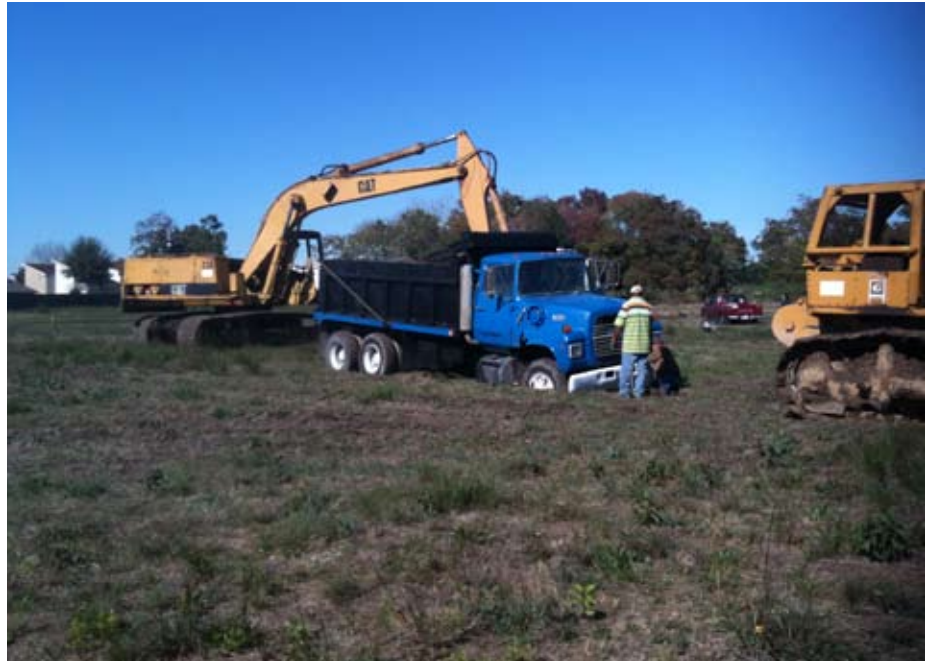
At one point, a dump truck had to be freed from the soft soil. Read on for more!
